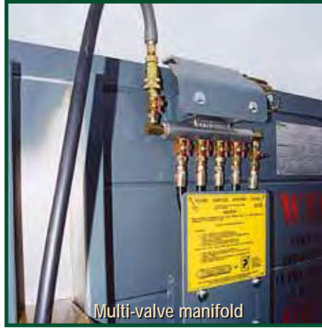
Pump can hose connection to manifold
